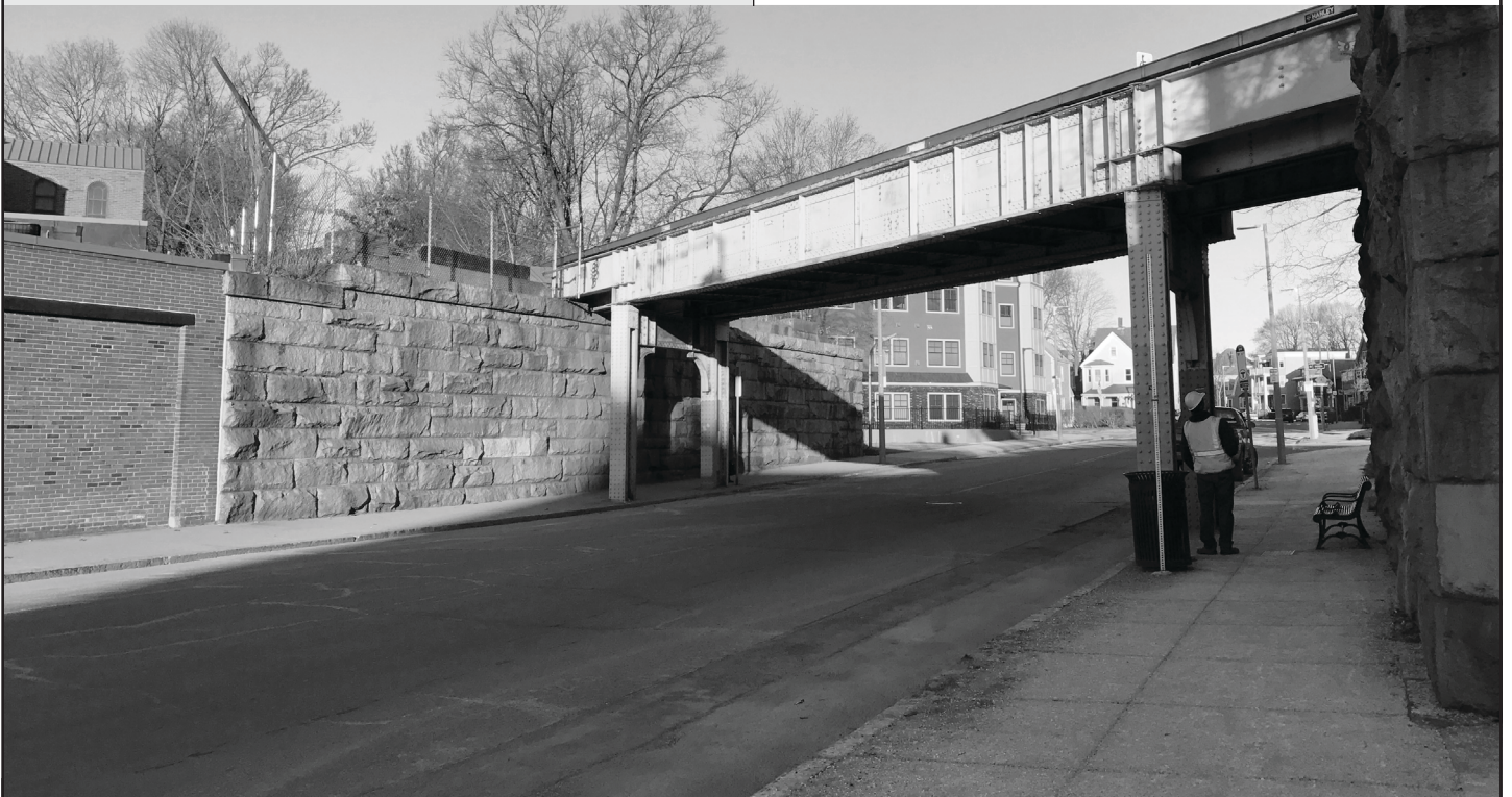
View of the MBTA-owned Commuter Rail bridge from Robert Street in Roslindale.
