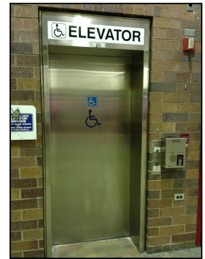
Elevator 805 at Red Line Lobby
