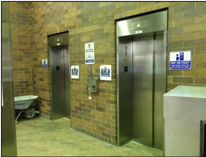
Elevators 806/807 at Garage Lobby to be Replaced
