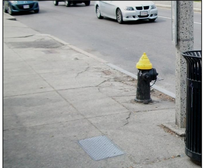
Broken Sidewalk at Boarding Area
