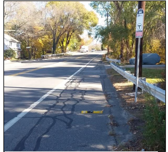
Inaccessible Bus Stop
