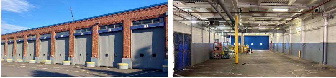
New overhead doors installed at the Everett Bus Facility and repainting at the Albany Bus Garage
