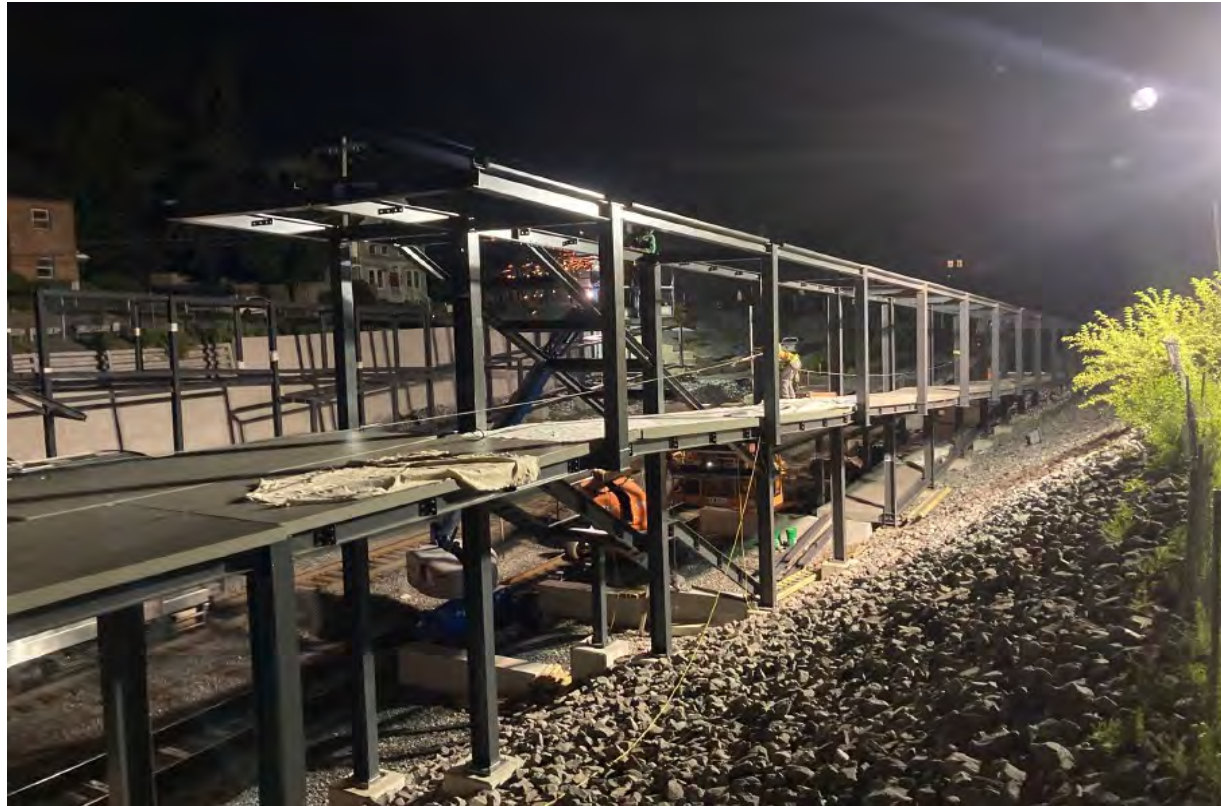
Inbound ramp: ramp welding and roof prep at East end of Station
