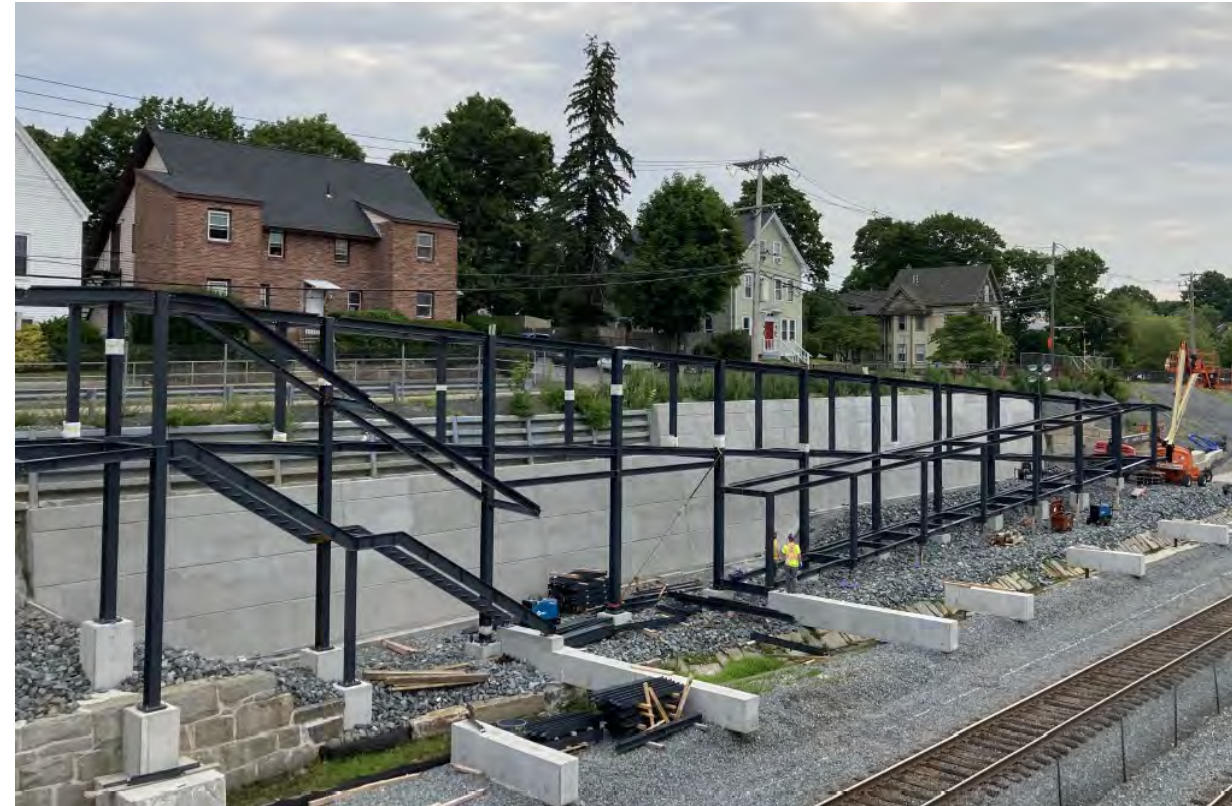
Outbound ramp: welding floor connections to ramp at East end of Station
