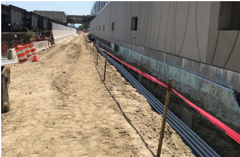
New fence installed on barrier (L) and duct bank (R) at East Access Road
