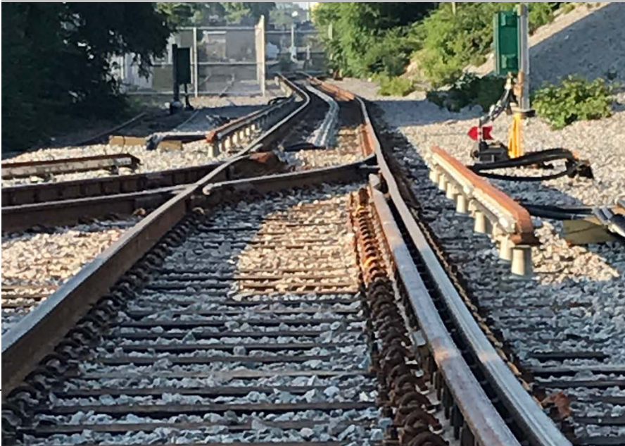
Installed Third Rail Insulators Leading into Turnout
