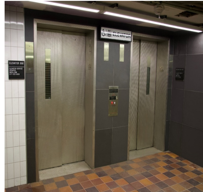
New DTX Elevator Nos. 998 and 999 at Orange Line Oak Grove Platform
